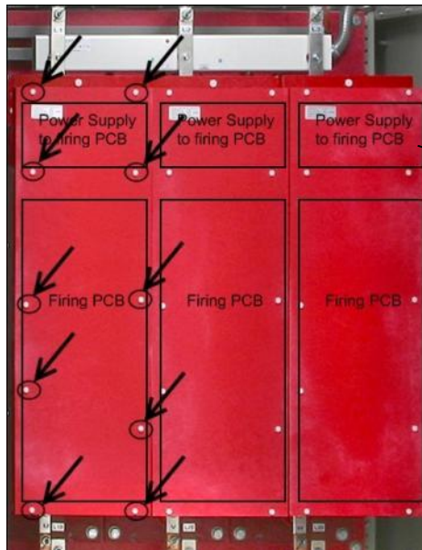
Front View of the Power Section
